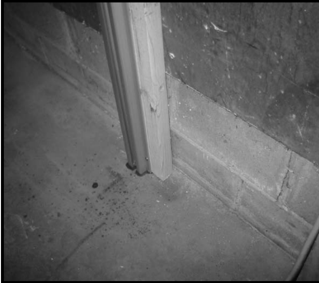
Extending 2x6 board to floor when installing to a tall masonry stem wall.
